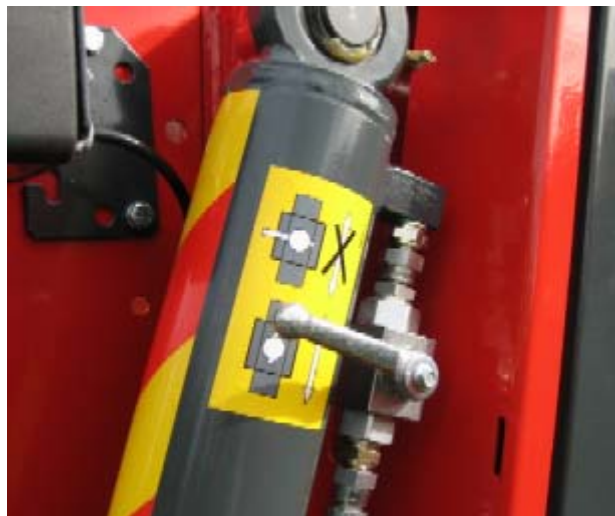
FIG. 20. Lifting cylinder safety valve closed
